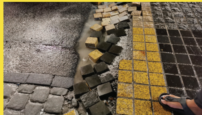
Picture 25: Temporary public works makes the surface unstable and unsafe, compromising walkability and public access.
