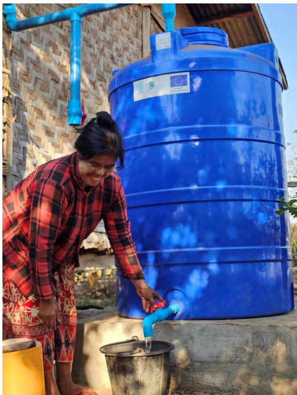
Figure 5(g). Household rainwater collection system.
