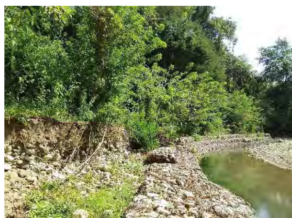
River gabions destroyed by flood in Bajak Village.
