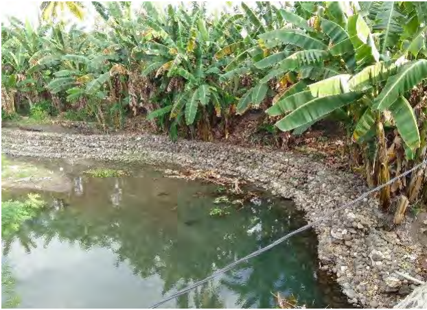
The river's gabion was destroyed due to a strong water current in Salama Village.
