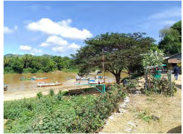
The Early Warning System (EWS) siren installed on the side of the Wae Pesi.
